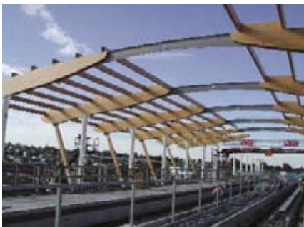
Architects connected spruce glulam beams, located on opposing platforms, with a steel flitch plate that arched across the light rail tracks.
