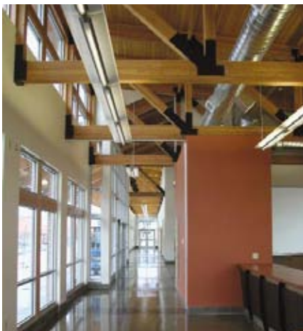
The station's interior was designed with exposed glulam trusses because the architect felt steel would be too harsh for the large public space.
