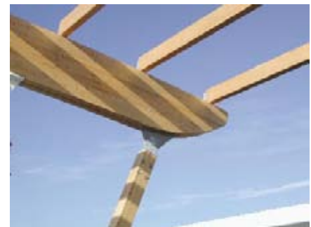
Glulam beams are connected to the supporting structure with concealed knife plates, kerfed into the beams, in Vancouver, BC's Rupert Station.
