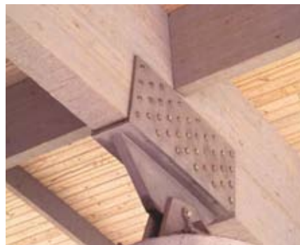
Large steel plates securely anchor glulam girders to the embedded anchor bolts in the concrete columns of the Indian Creek Station in Atlanta.
